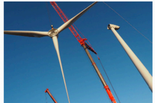
Wind Turbine at Alvington Court
