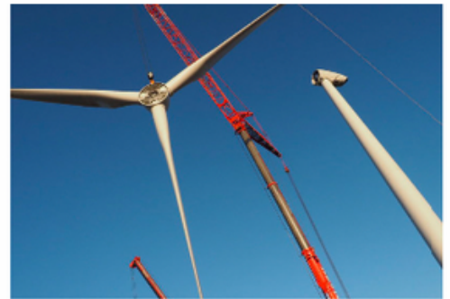
Wind Turbine at Alvington Court
